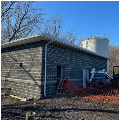
The booster station and water tower storage tank in Rahmer Park as of December 2022.
