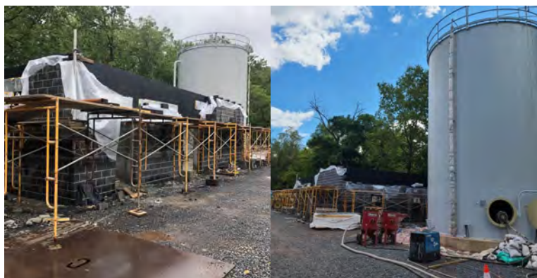
The images to the left portray the construction of the booster station in Rahmer Park.
